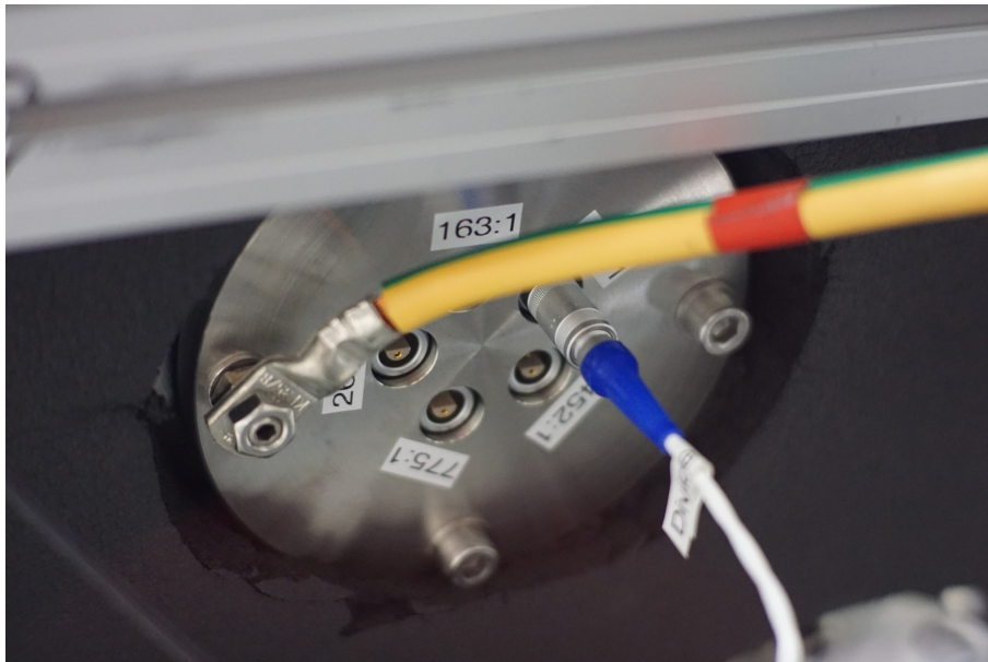
Figure 1: Tap flange with grounding cable and output cable attached.
